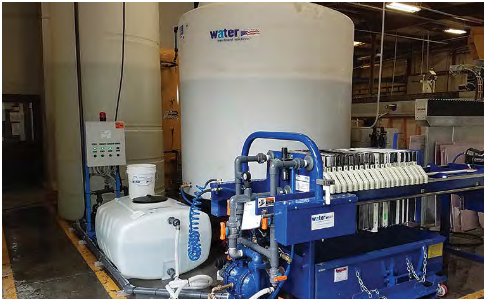
Photo Courtesy of Water Treatment Solutions
